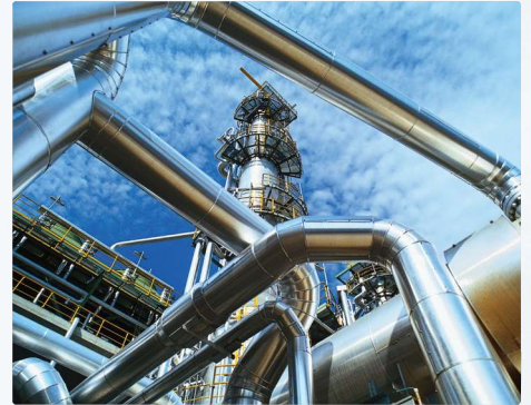
Chemical, Oil and Gas
